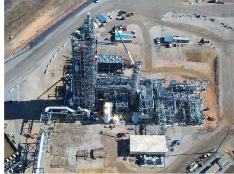
MHI's KM-CDR Process at Plant Barry Property of MHI and/or Southern
