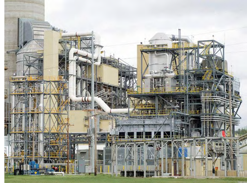
Alstom's Chilled Ammonia Process at AEP's Mountaineer Property of Alstom Power and/or AEP
